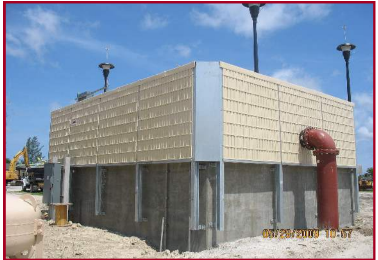
Retrofitted LSE Absorptive Pump Enclosure
