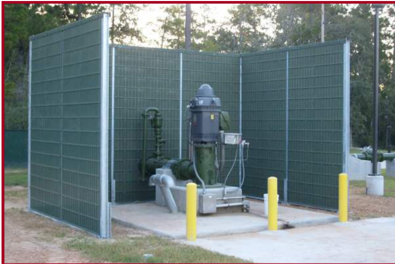
3-Sided LSE Absorptive Pump Enclosure
