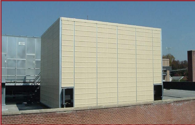
LSE Absorptive Rooftop Enclosure
